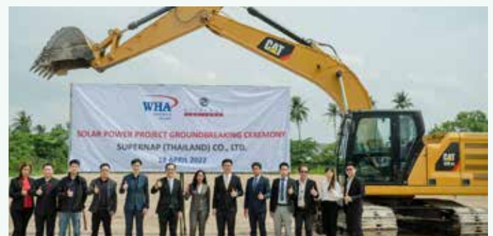
In the picture: Dr. Niphon Bundechanan (center left), Former CEO of WHA Utilities and Power PLC, together with Mrs. Sunita Bottse (center), Chief Executive Officer of SUPERNAP (Thailand) Co., Ltd., held a groundbreaking ceremony to start the construction of SUPERNAP Thailand's solar farm project, which will cover 10,000 sq.m. of space.
